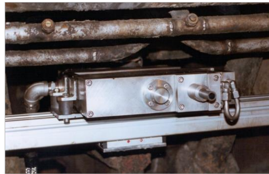
Figure 1: On-line work roll inspection system in stand F2 at ArcelorMittal Gent
