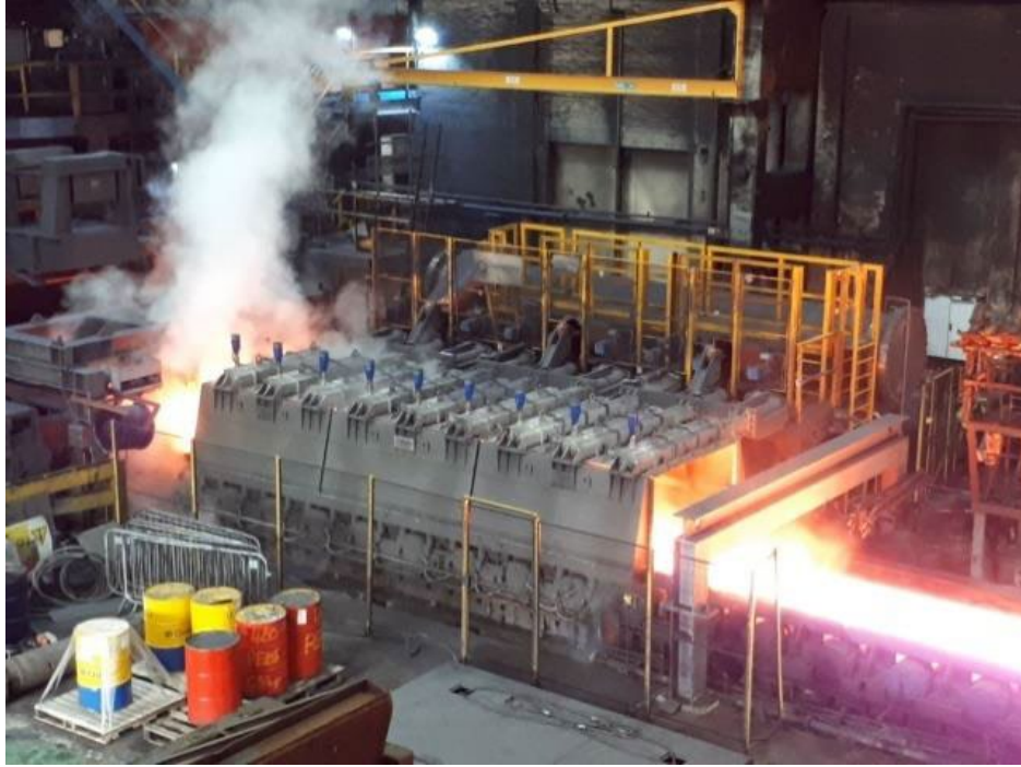
Figure 1: Transfer bar cooling system installed at the hot strip mill of Tata Steel's Port Talbot [2].
